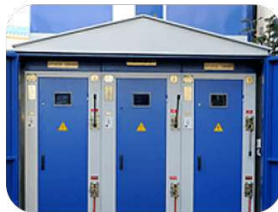
Transformers ( Ural transformer plant LLP )
