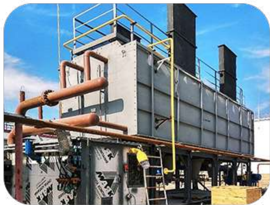
Oil heating furnaces ( "WKMK" JSC )
